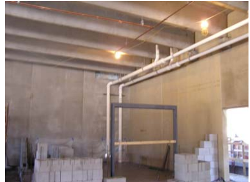
Interior of the new Hatcher WTP
